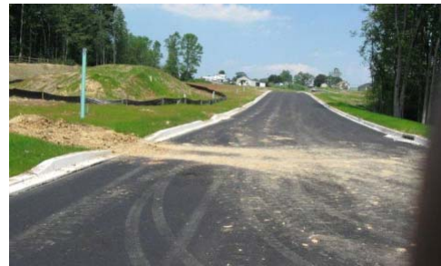
Illegal vehicular tracking of sediment onto public road
