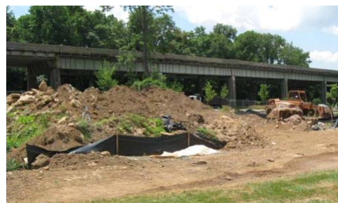
This silt fence needs to be completely reinstalled and maintained
