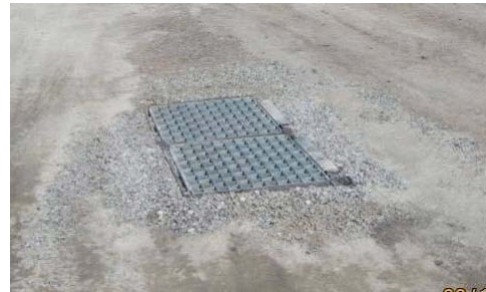
Inlet has no inlet protection. Protection must be
