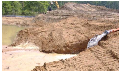
All dewatering practices require approved filtering devices. This outlet has completely washed out
