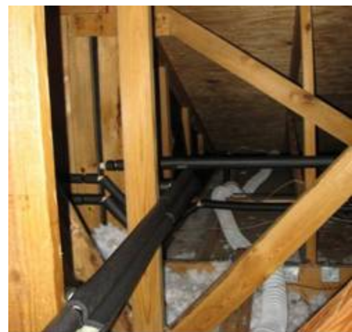
Figure 3: Insulated CPVC lines
